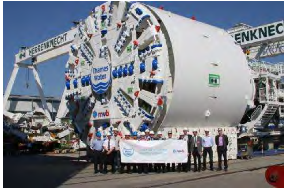
TBM Factory Test Visit May 2011
